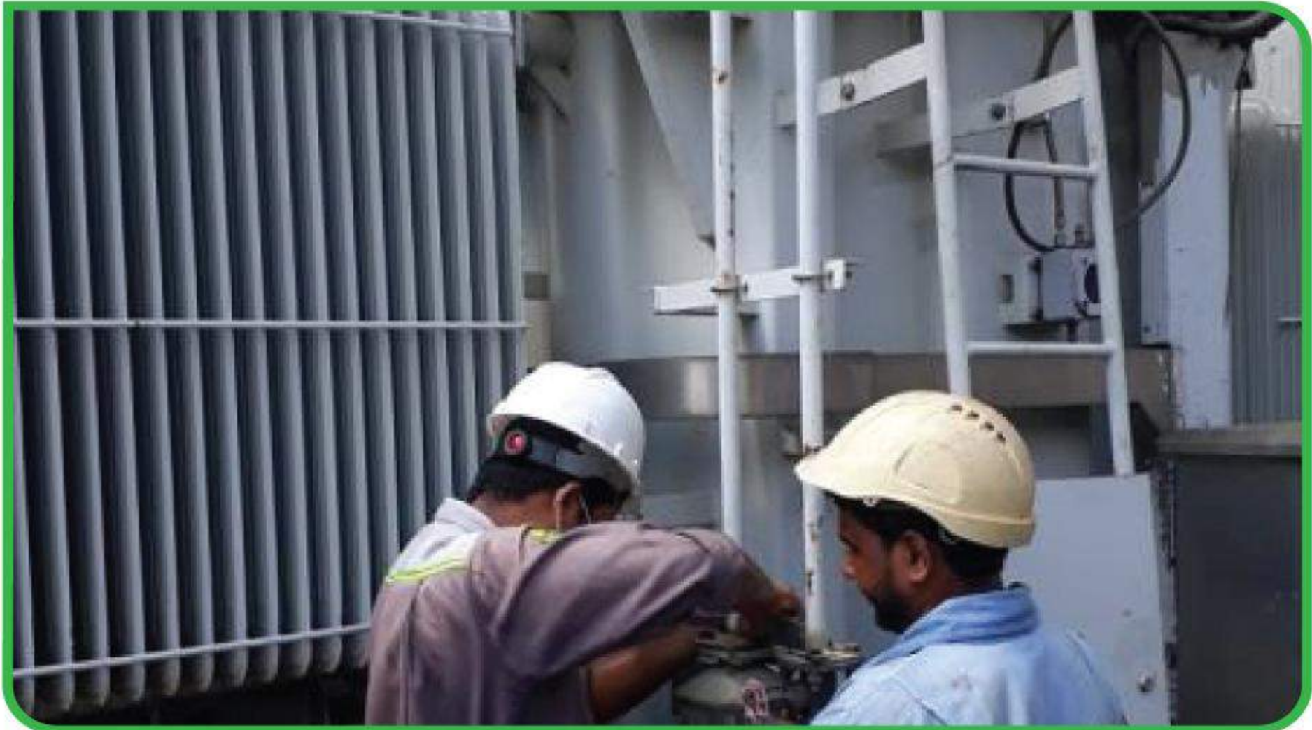
Changing of Transformer Silica Gel at Raozan 25 MW Dual Fuel Power Plant, Noapara, Raozan, Chattogram.
