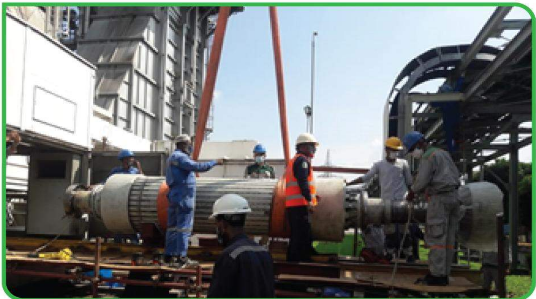
Major maintenance work of Rotor of Mymensingh 210 MW Combined Cycle Power Station, Shambhuganj, Mymensingh.
