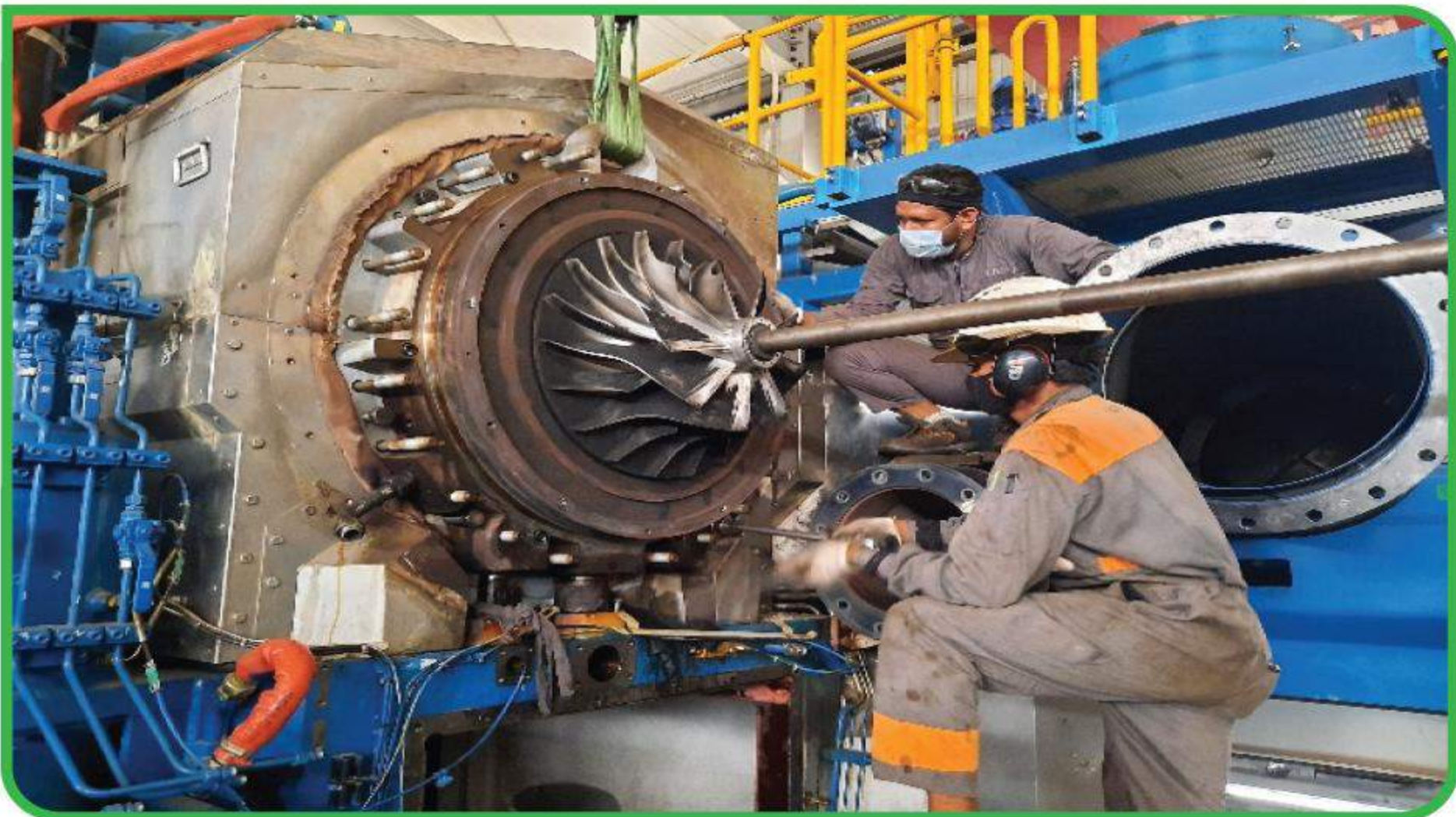
Scheduled maintenance of Engine Turbocharger at Gazipur 105 MW HFO Engine based Power Station, Kadda, Gazipur.
